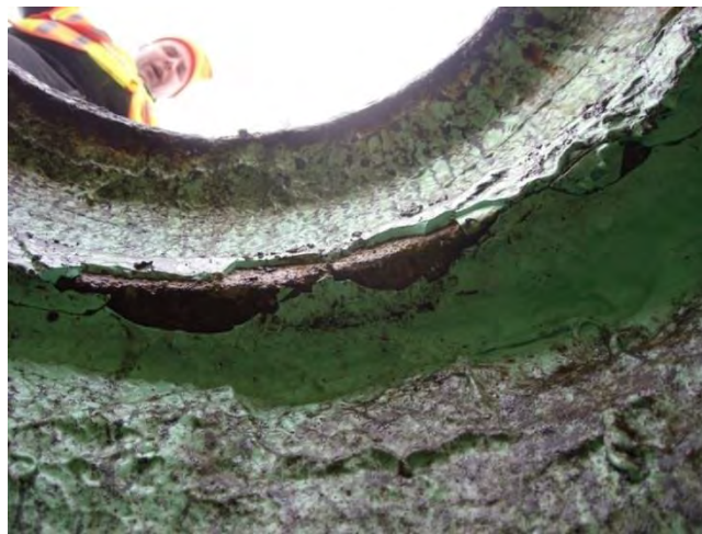
Figure 6-2. Polymeric Liner Failure Along the Edges Inside the Manhole.
