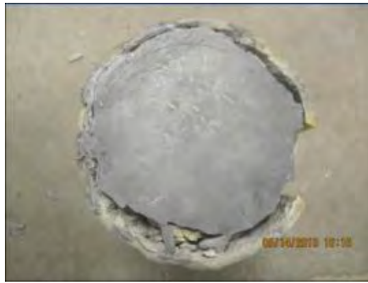
Figure C-43. Liner Detachment from the Concrete Substrate (PU-C#5).
