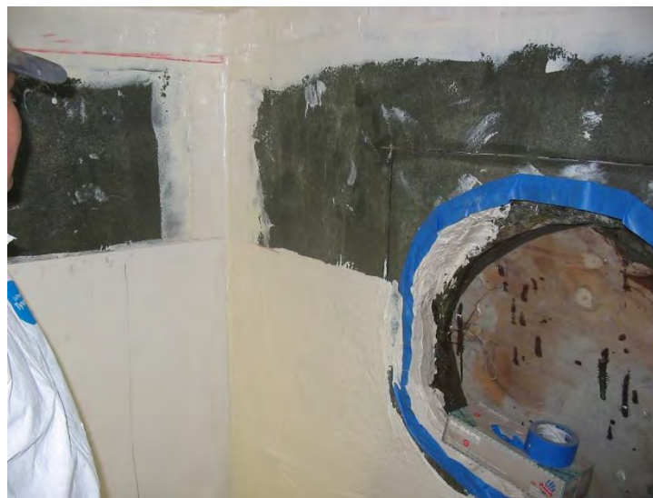
Figure 6-17. Two-Part (Extruded PVC Plus Cured-in-Place Polymer) Being Applied at the Junction Chamber.
