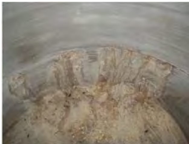
Figure 6-6. Cementitious Liner that Experienced Material Sloughing.
