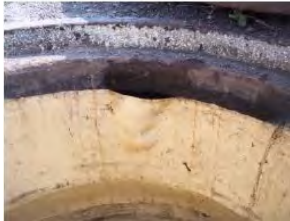
Figure 6-7. Spray Applied Liner that Peeled Away from the Substrate.
