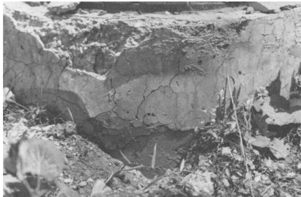
Figure 2-3. Example of Severely Deteriorated Manhole Cone Investigated in the Cady and Weyers Study.
