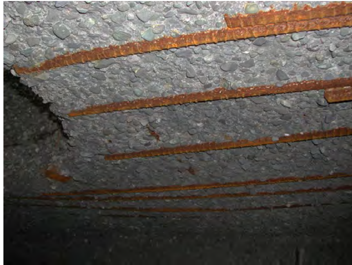
Figure 6-16. Junction Chamber Prior to Rehabilitation. Note the Severe H 2 S Induced Corrosion.
