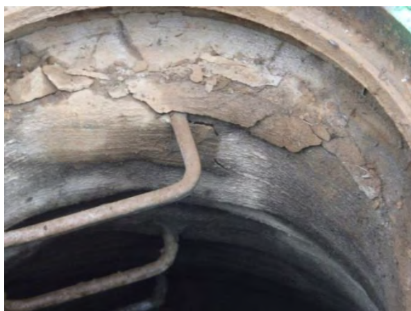
Figure 6-22. Cracking in the Fiber-Reinforced Cement Liner Within a Few Years of Installation.
