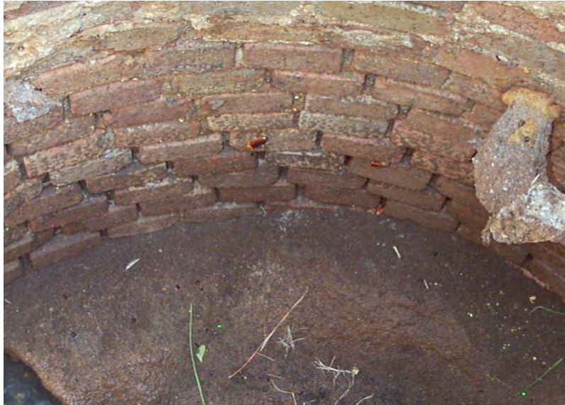
Figure 6-4. Wall Condition Deteriorated (Heavy).
