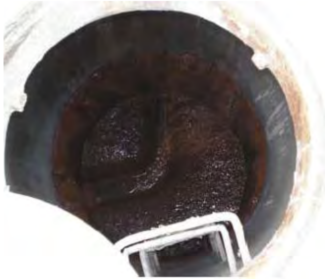
Figure 6-9. Infiltration (Runner) Along the Joints.
