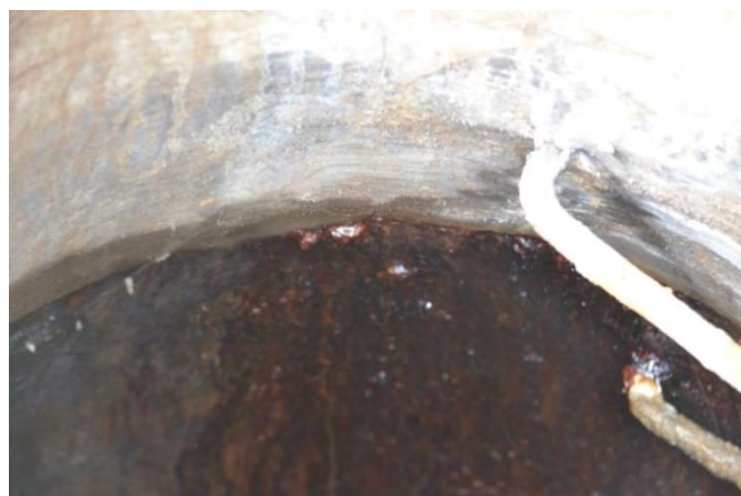
Figure 6-23. Infiltration/Inflow Marks Due to Cracking in the Fiber-Reinforced Cement Liner Within a Few Years of Installation.
