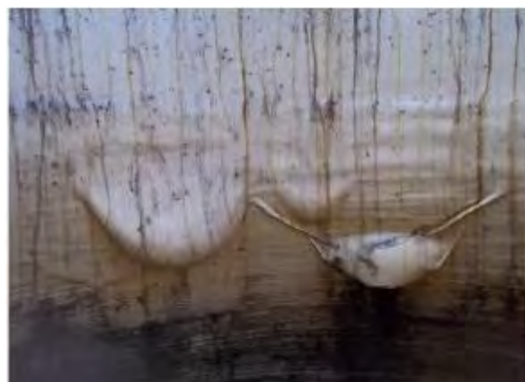
Figure 6-8. Spray Applied Liner that Exhibited Bubbles.
