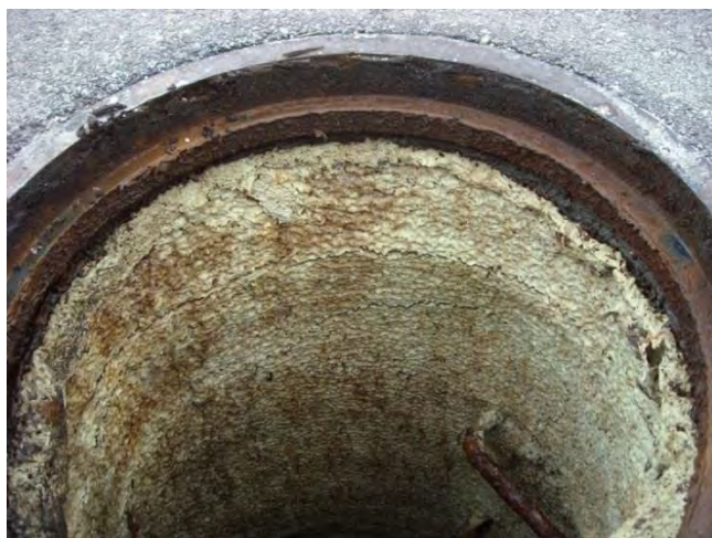
Figure 6-1. Blistering and Pitting Observed on a Composite Lining System. (Cement Lining and Polymer Coating on Top)
