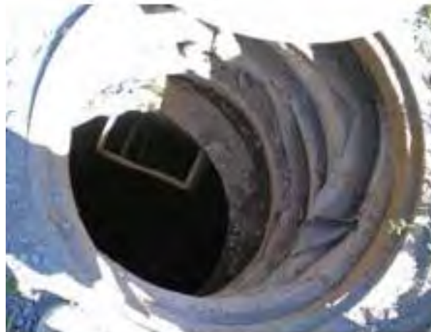
Figure 6-12. Misaligned Grade Rings.
