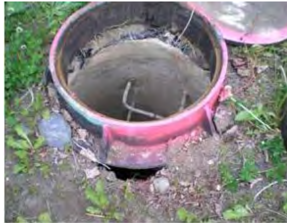
Figure 6-11. Shifted Manhole Frame with a Gap.
