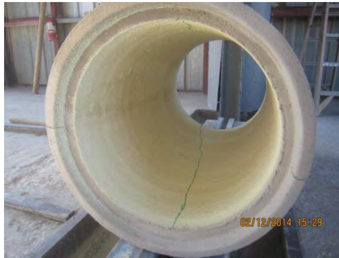
Figure 4-21. Example of Simultaneous Cracking in the Concrete Substrate and Liner.
