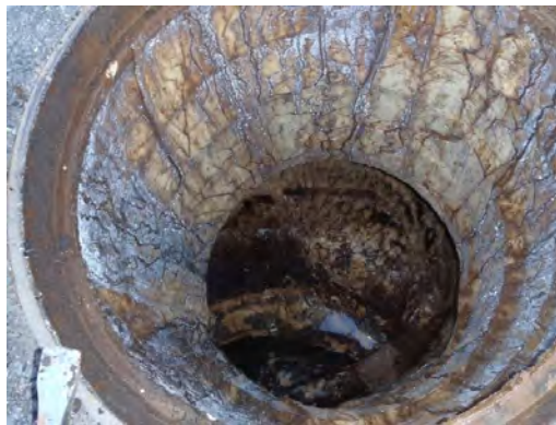
Figure 6-5. Manhole That Was Lined (Cured-in-Place) with Reinforced Polymeric Lining. The Liner Seems Intact after 13 Years of Service with No Apparent Defects.
