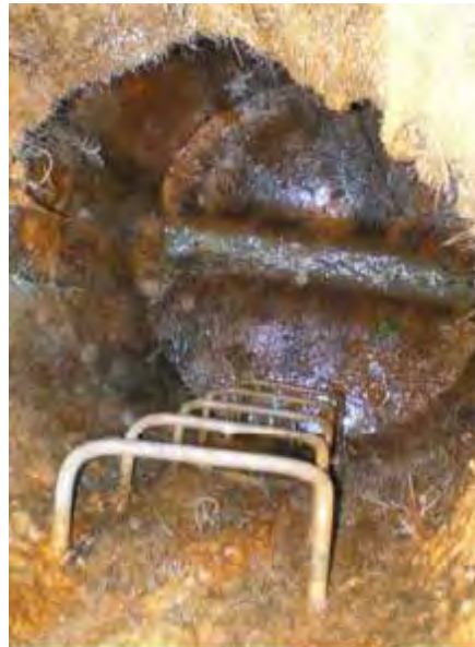
Figure 6-10. Manhole with Heavy Root Intrusion.
