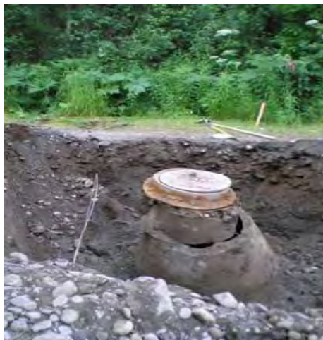
Figure 6-14. Manhole with Broken Cone.
