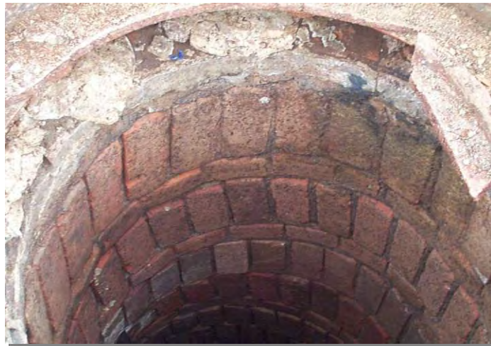
Figure 6-3. Corbel Condition Deteriorated.
