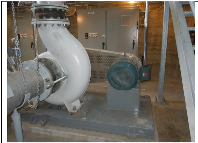
Figure 4a : Jet pump is used to mix the biosolids, control foam, and distribute oxygen in the biosolids.
