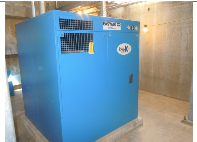
Figure 4b: Blower to supply oxygen to the SNDR unit
