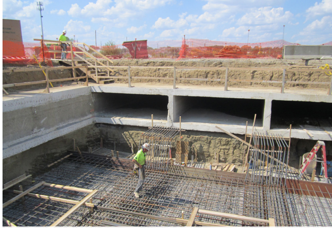
Combined Sewer Pump Station, Fort Wayne, Indiana
