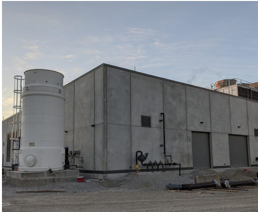
Marion County Justice Center Campus Central Utilities Plant, Marion County, Indiana
